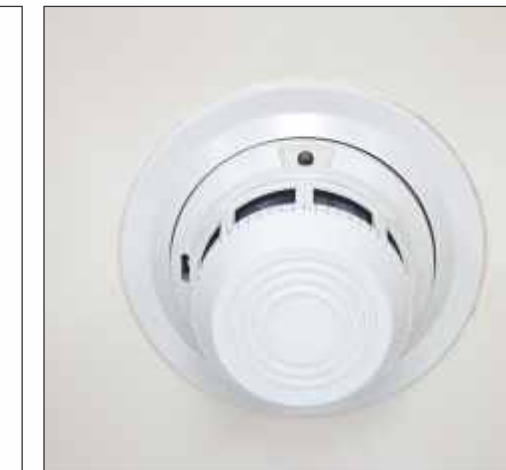
Smoke Detector With Automatic Fire Fighting System
